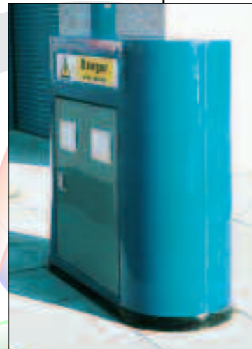
MR2 - TELECOMMUNICATIONS EQUIPMENT
