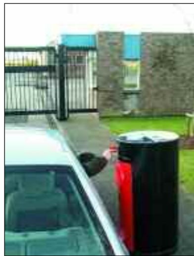
MR3 - GATE SECURITY SYSTEM
